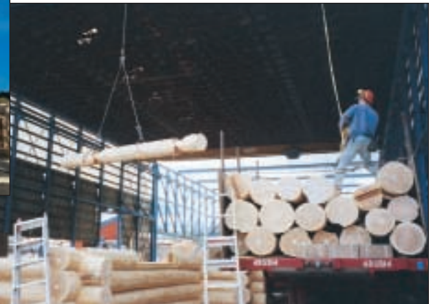
Upon completion of the log shell in our construction yard, the home is re-inspected for quality and it is number coded and loaded for shipment.
